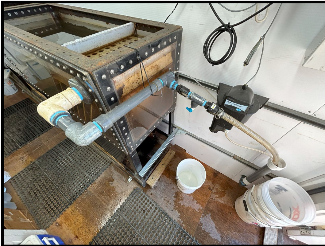
Figure 6: IPS Effluent Piping
