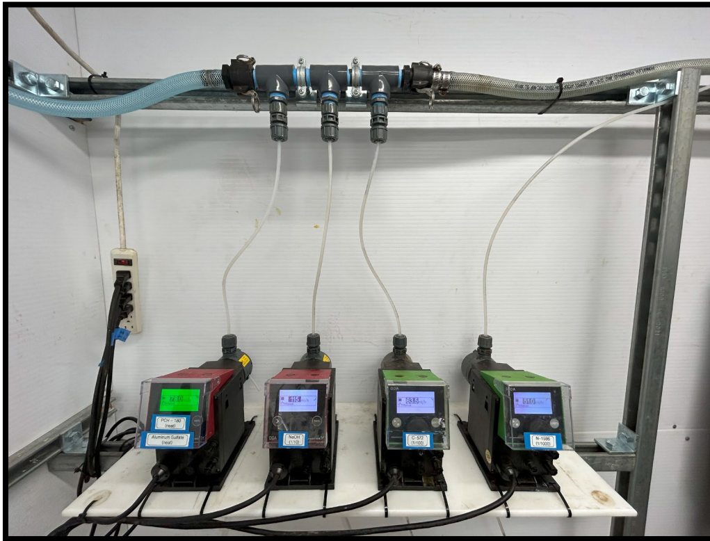
Figure 2: IPS Chemical Feed Pumps
