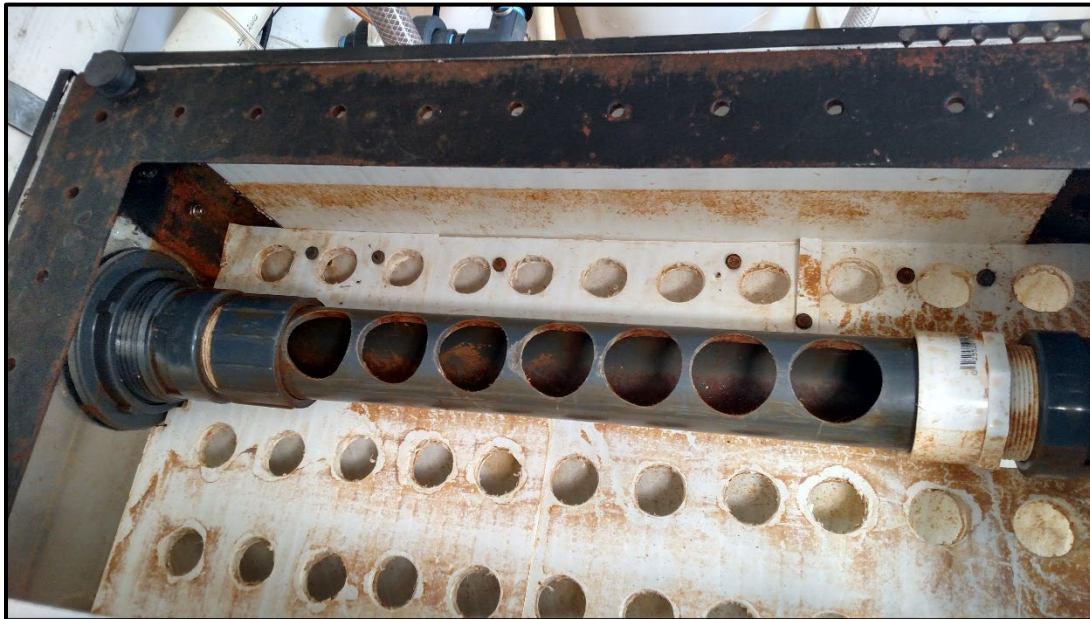
Figure 5: Top Plate and Effluent Weir on IPS
