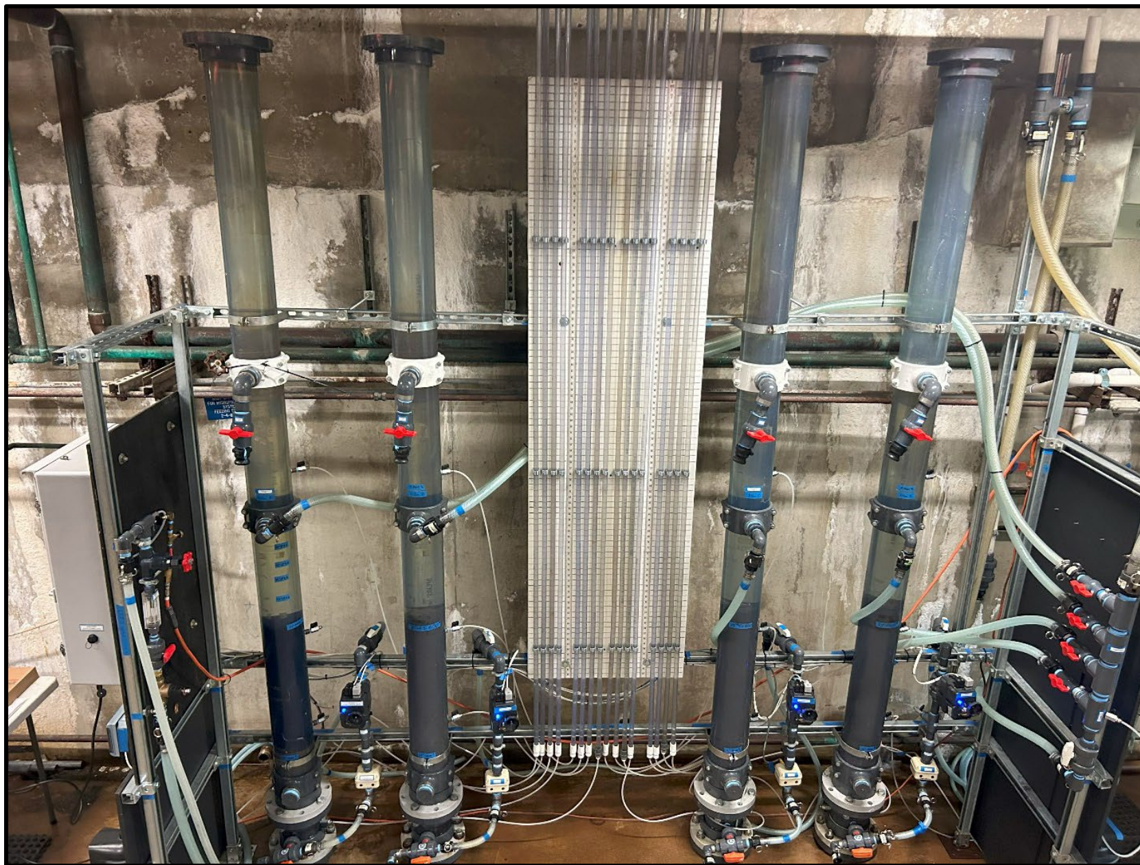
Figure 7: Pilot Filters with Four Filters (two filter proposed for Ellsworth)
